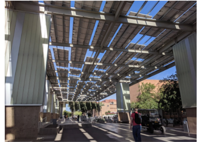
Solar PV Walkway @ Arizona State
